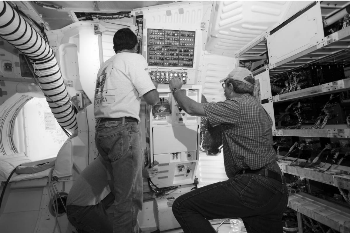
Figure No. A-23. Installation of the shuttle orbiter repackaged galley into Discovery's middeck. The galley was removed following Discovery's last mission, and sent to Houston, where it was cleaned and deserviced by USA as part of the shuttle transition and retirement efforts, November 15, 2011.
