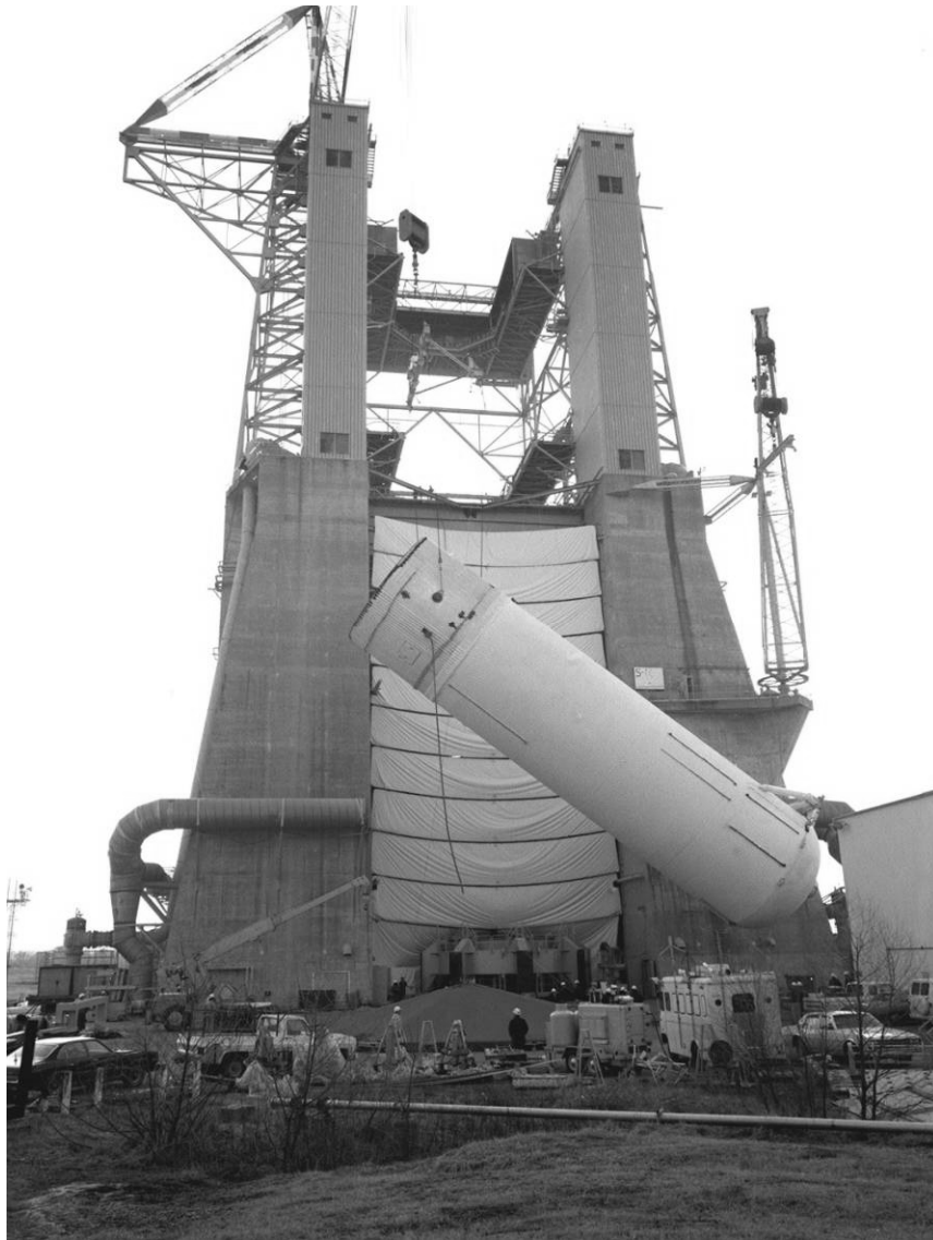
Figure D-1. Liquid hydrogen tank of the ET is installed into the S-1C Test Stand at MSFC for a structural test, March 1, 1978.
